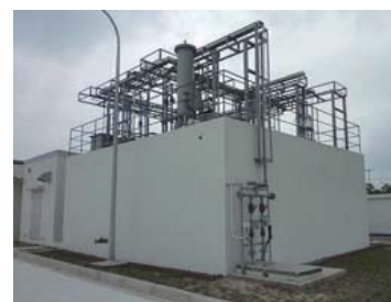
Wastewater treatment facility (BMV)
