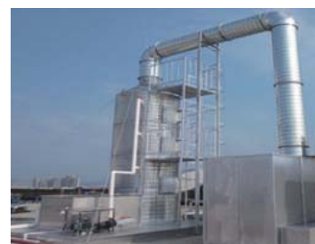
VOC treatment facility (BTSL)
