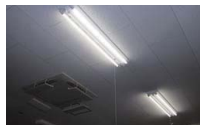
LED fluorescent lamps and canopy switches
