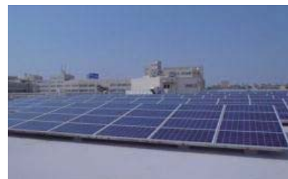
Photovoltaic power generation system expanded at the Mizuho Manufacturing Facility
