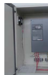
Inverter control console
