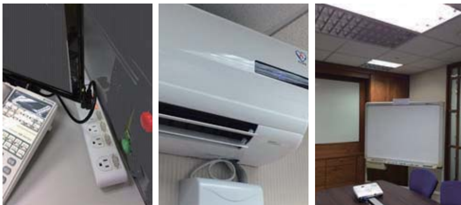
Independent switches were added to reduce power consumption. The temperature settings of air-conditioning equipment were reviewed. Lights were switched off and removed whenever and wherever unnecessary.
