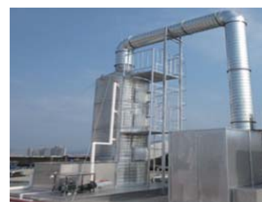
VOC treatment facility (BTSL)
