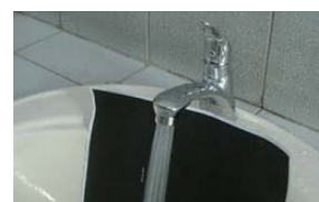
Faucet after taking water-saving measures
