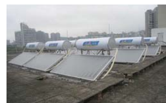
Solar water heater
