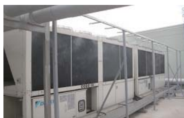
Water spraying on outdoor units
