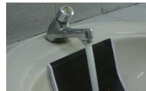
Faucet before taking water-saving measures
