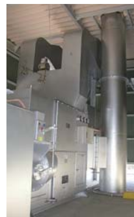
Catalytic combustion facility
