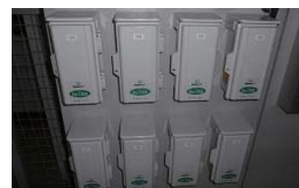
Energy conservation control system
