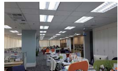
LED lights used in the office and service center
