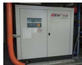
Newly introduced air compressor (inverter-driven)
