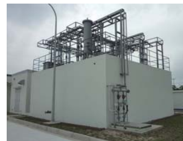
Wastewater treatment facility (Brother Machinery Vietnam)
