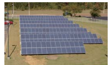
Photovoltaic power generation systems set up at two locations
