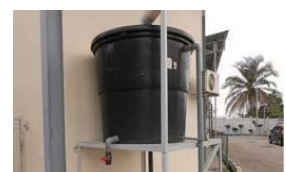
Rainwater storage tank (Brother Industries Technology (M) Sdn. Bhd.)
